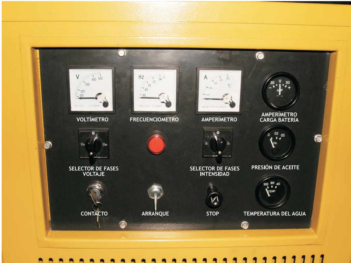
PANEL DE CONTROL Fig. 1
